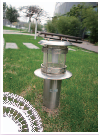
Solar Light installed in public area, which can make useful of natural energy for lighting.
