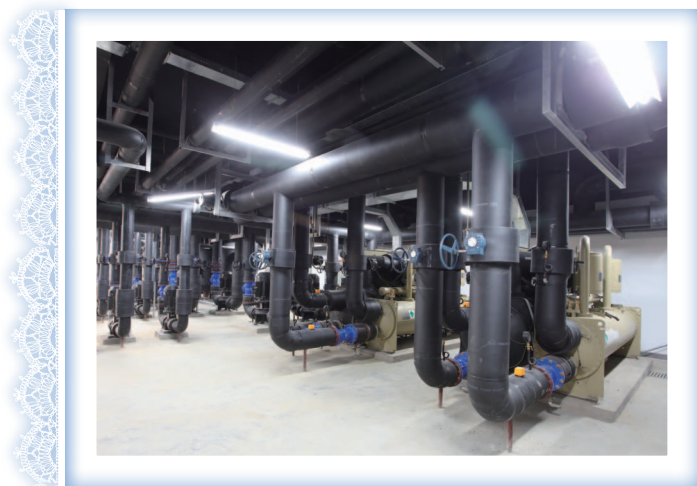
A geothermal heat pump air conditioning system in Shandong plant
